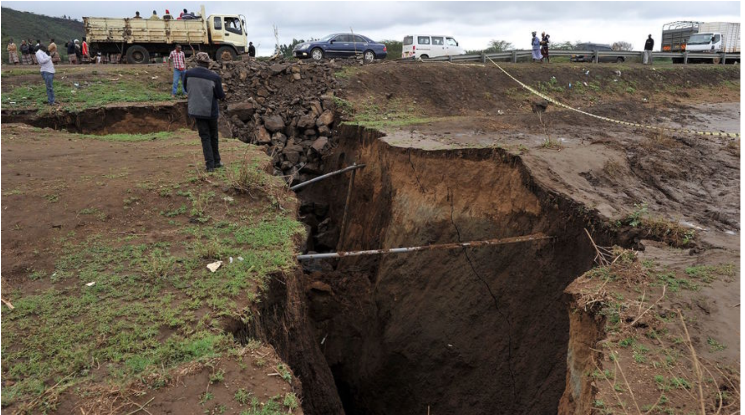
Image 1. Vehicles drive next to a deep split on a repaired road that had been washed away during a heavy downpour at Maai-Mahiu, Kenya, on March 15, 2018. Photo by: Tony Karumba, AFP/Getty Images
